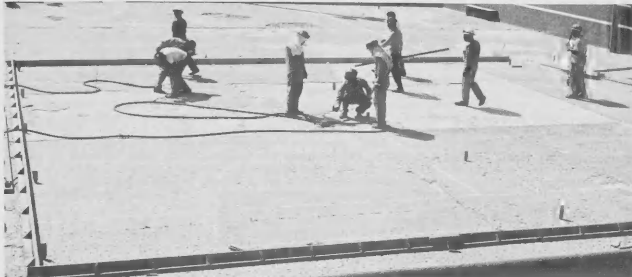
LAGO WORKMEN assigned to the Lago Sport Park project are shown assembling screeds, or the lengths of board which are set at the desired height and then used as guides to level the concrete as it is poured.
